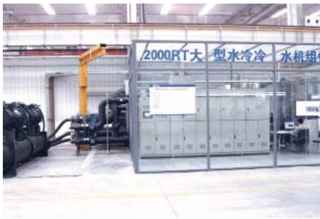
2000RT Water-cooled Chiller Test Lab
